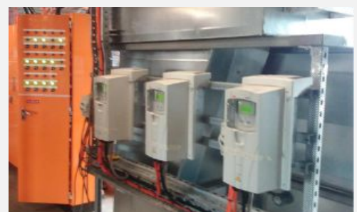
Variable speed drives installed on HVACs
