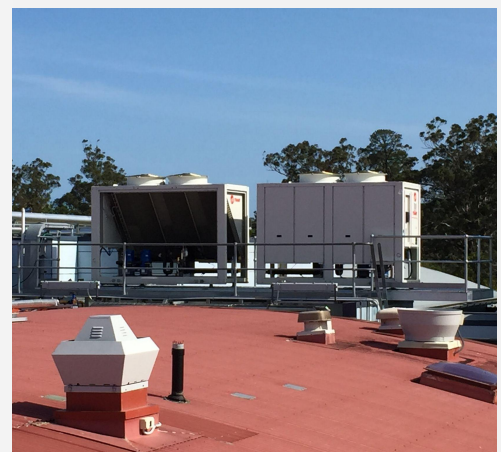
Updated HVAC systems installed
