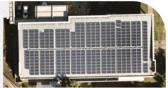
Solar photovoltaic panels installed on site rooftops
