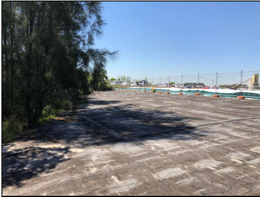
Photo 5: Area outside northern site boundary showing barrier installed as part of remediation work under previous Council consent.
