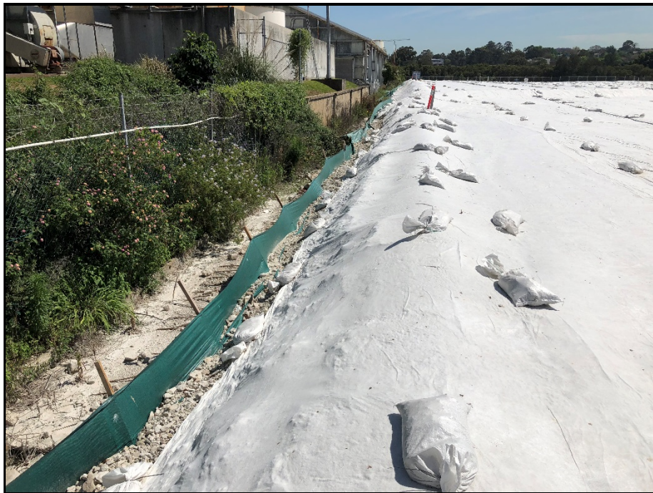
Photo 6: Western site boundary showing weeds encroaching from neighbouring site.
