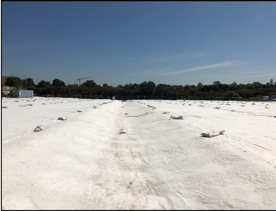
Photo 1: Geofabric over preloading material. Looking north towards Parramatta River from centre of site.
