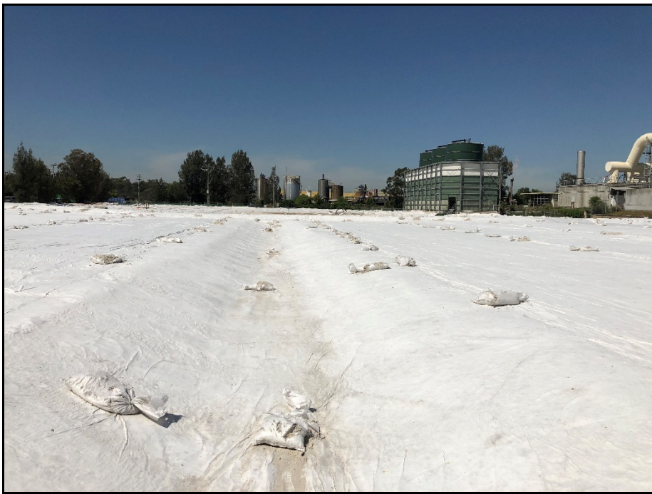
Photo 2: Looking south towards Grand Avenue from centre of site. Tanks remaining in south western corner to the right of the photo.
