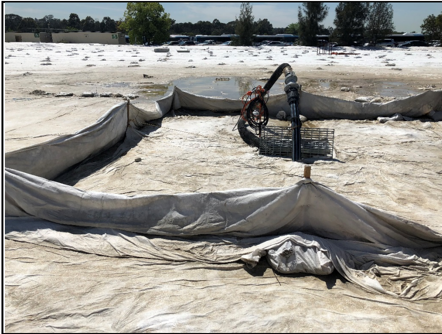
Photo 3: Temporary stormwater sump at southern end of the site.
