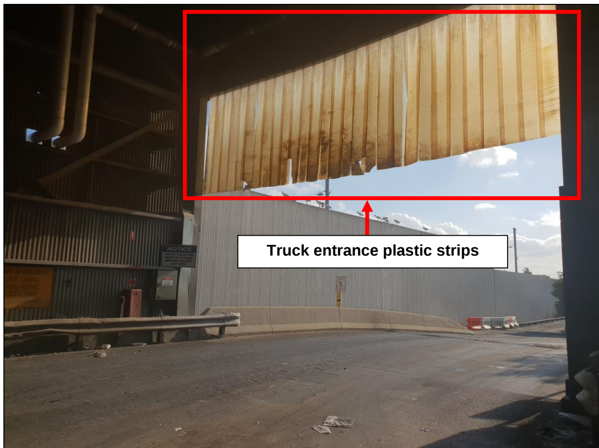
Photo 2.4 –Truck entrance plastic strips as found on 24 May 2018
