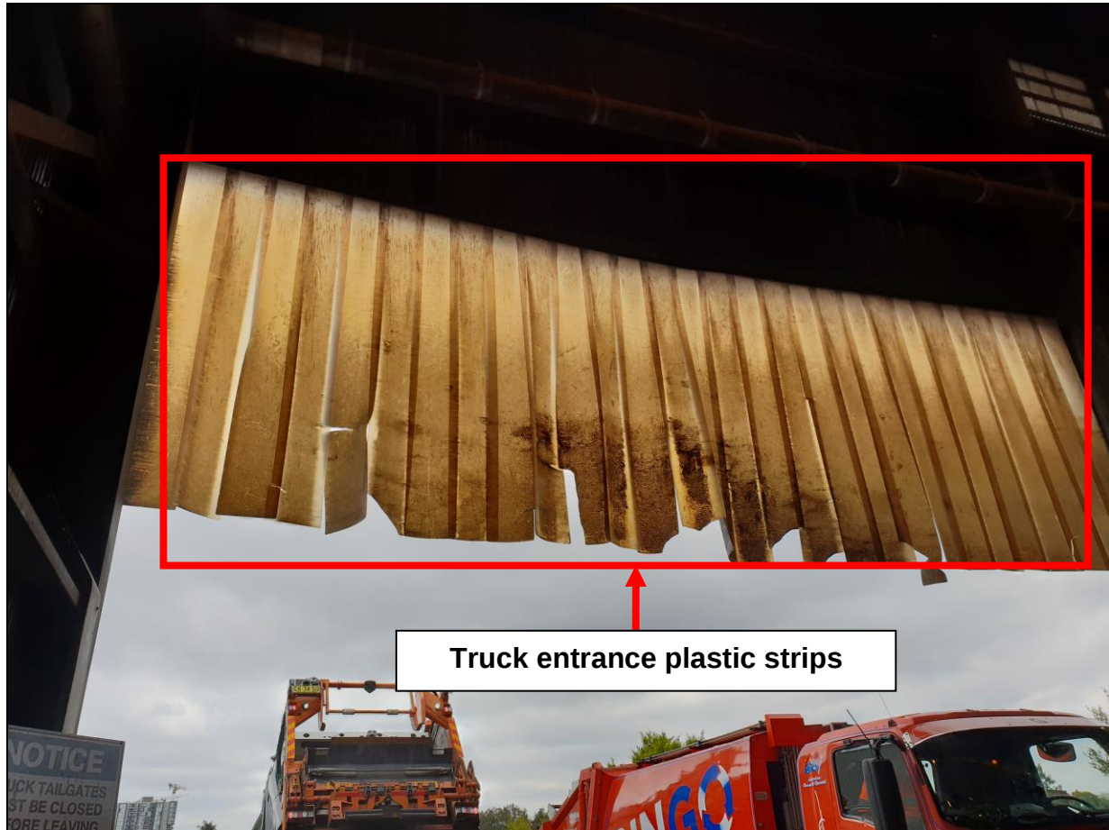
Photo 2.4 –Truck entrance plastic strips as found on 15 November 2018
